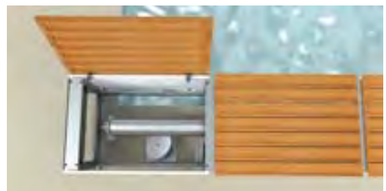
Access to the skimmers and mechanical parts
